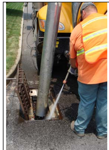
Cleaning out an inlet with the Jet Vac. Photo by Ocean County Engineering Department.
